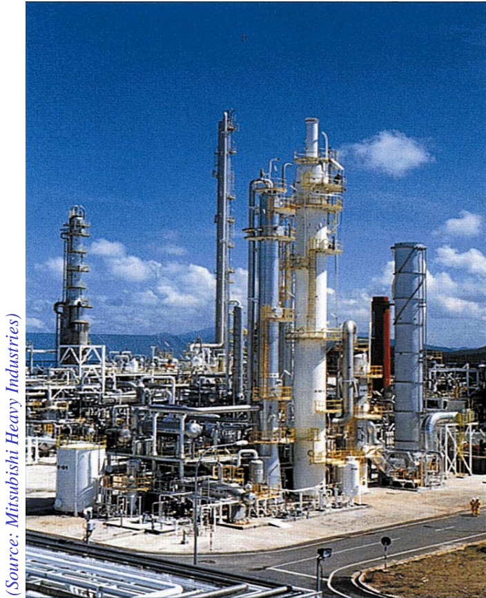
Post-Combustion Capture ( gas-fired power plant, Malaysia )
